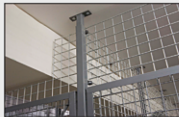
cut-outs around vents
